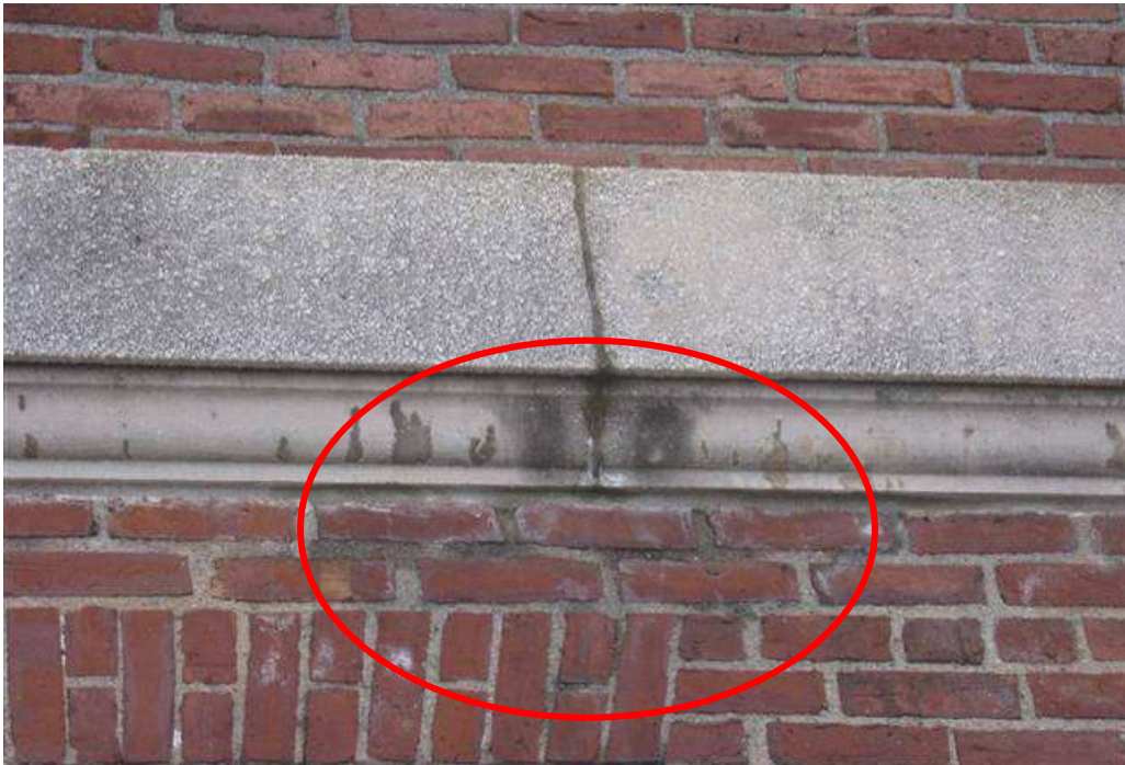
Spalling mortar joints
