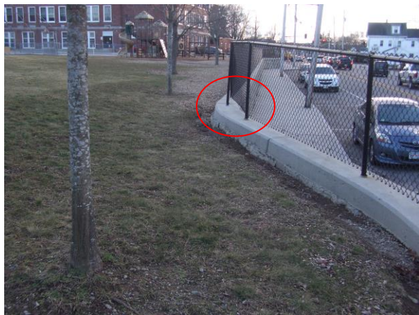
Fence on retaining wall, fabric pulling away
