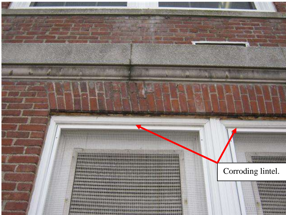
Visible lintel corrosion
