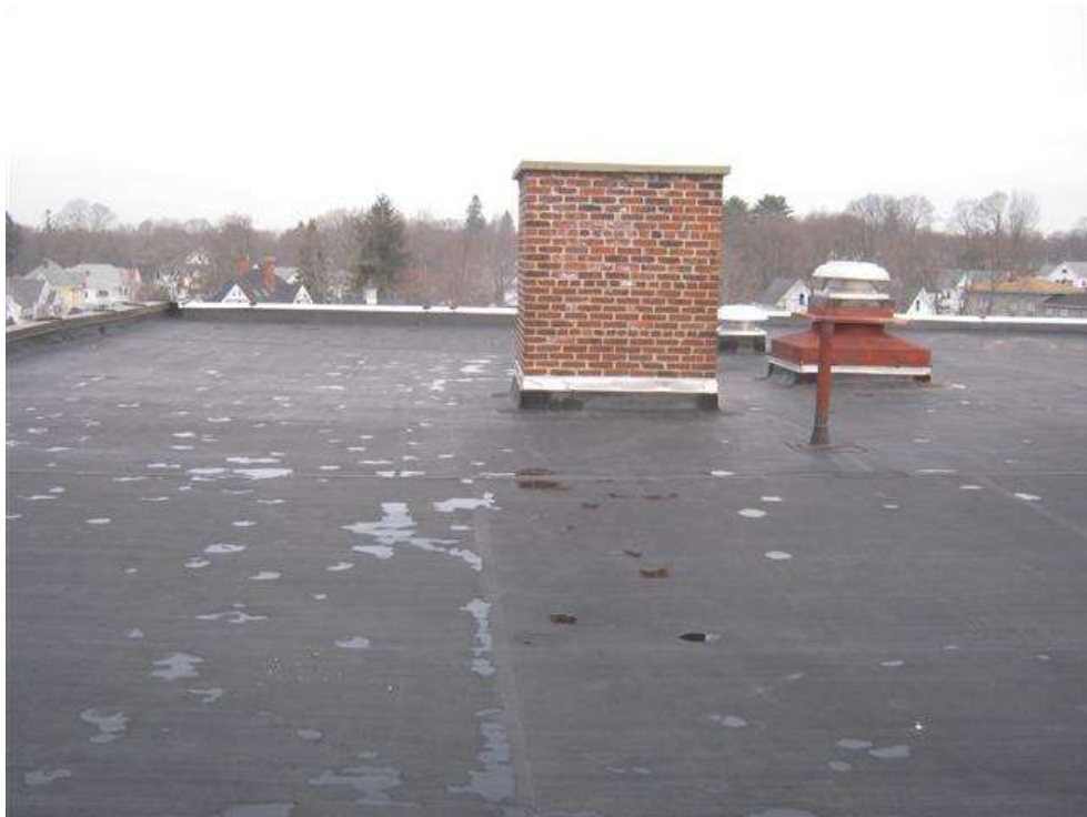
Spalling and cracking in chimney brick and cap looking north
