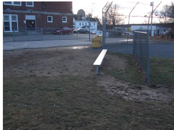
Low area retaining water, turning to mud
