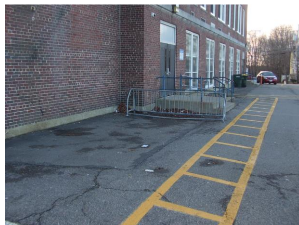
Patching and cracking north of the school
