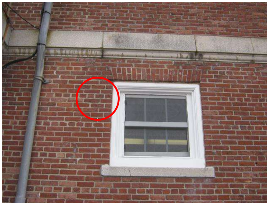
Spalled mortar joint at steel lintel
