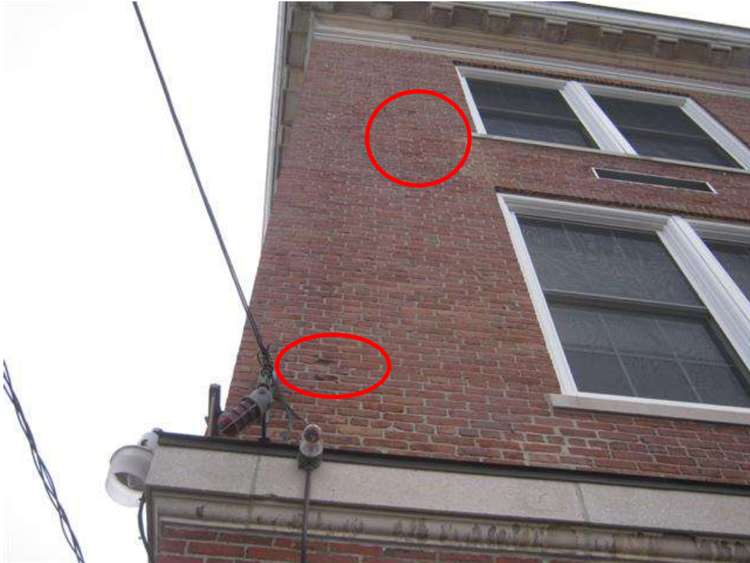
Spalling brick face
