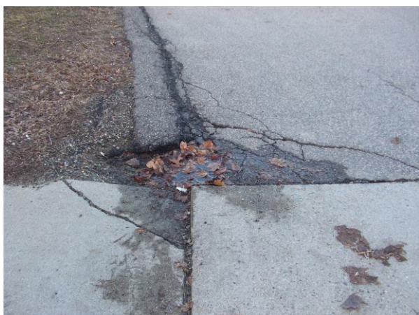
Water damage at Rte. 140
