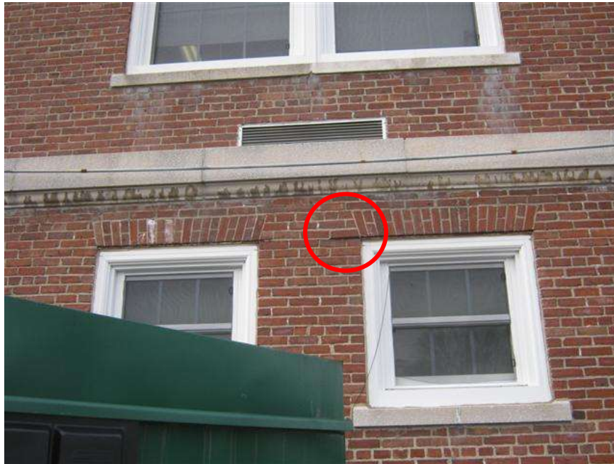
Spalled mortar at lintel bearing condition
