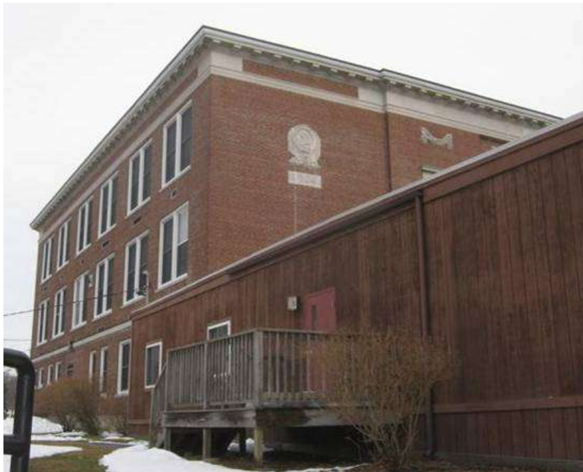
Portable classrooms with deteriorating sheathing along the west face
