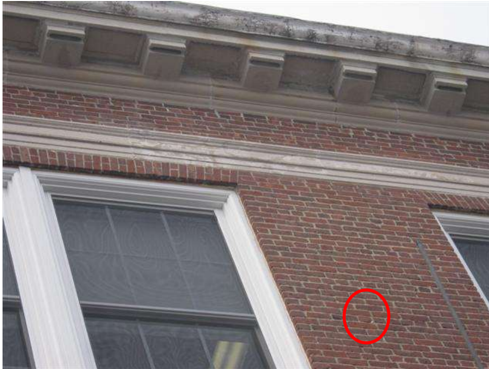
Isolated spalled brick faces
