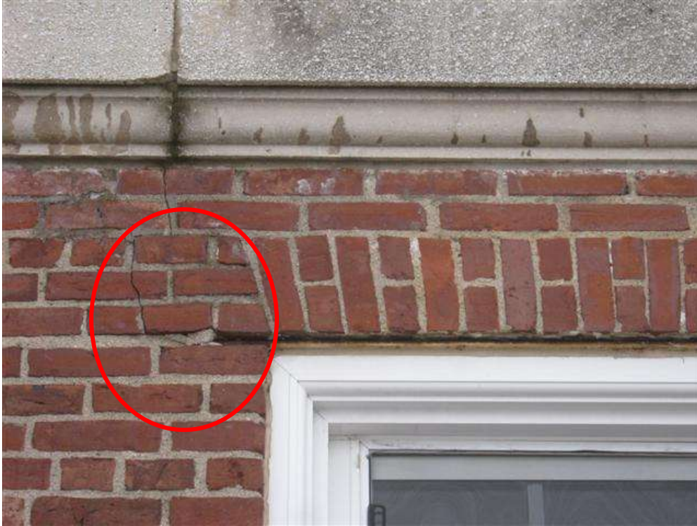
Close up of spalling and cracking brick indicating movement in the lintel due to corrosion
