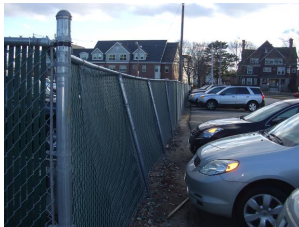
Fence bent out of place/ Dean College property line
