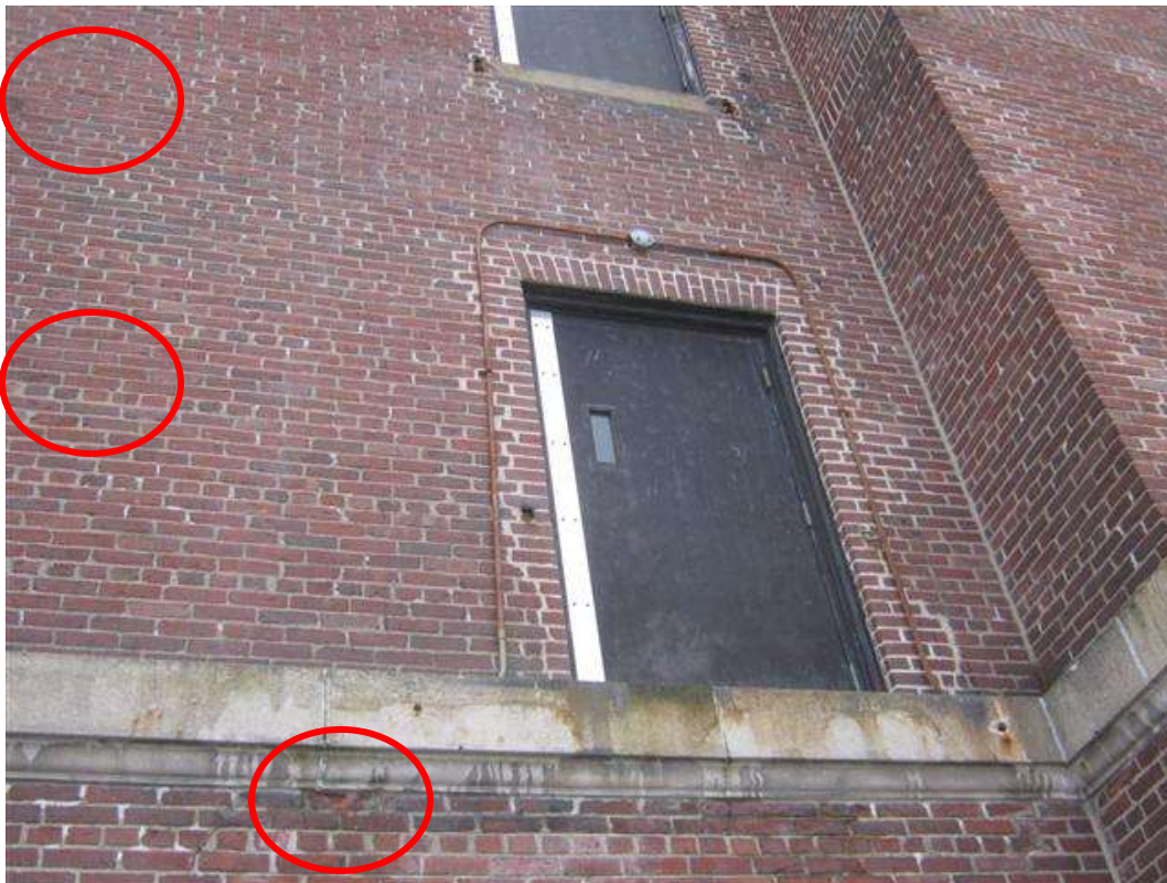
Isolated spalling brick on north face of building
