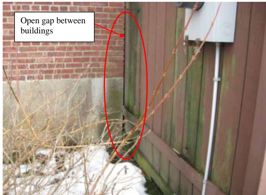
Sheathing turning green due to constant wetting
