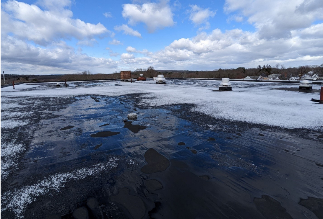
Figure 11 – Photo showing roof properly pitched to roof drains, and limited roof top equipment.
