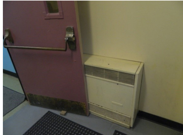
Typical Cabinet Unit Heater
