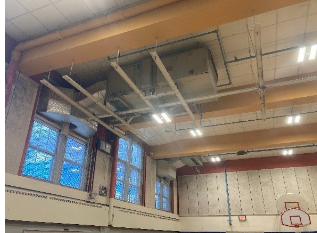
AHU-2 at gym ceiling & horiz. UV beyond
