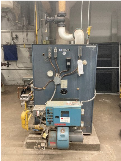
Boiler, Front View
