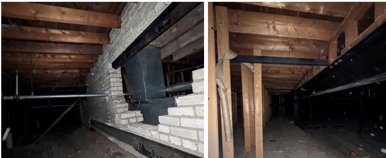
Figure 10 – Steel truss roof framing over library area, and cripple walls providing pitched roof construction.
