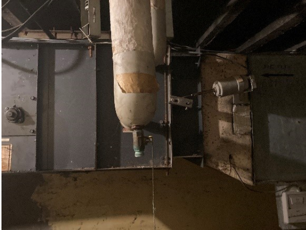
AHU-1 in basement, note pneumatic actuator
