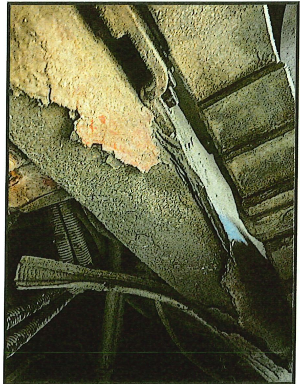
Drivers Side Frame Rail Showing Extreme Delamination
